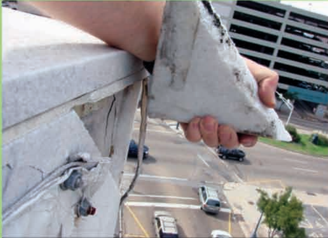
Spalling of a marble cladding caused by building movement.
