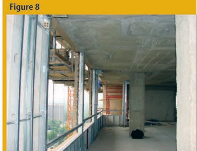
The slender brick pier located at the mid-span of this cantilevered slab may find itself sharing the load and ultimately failing.
