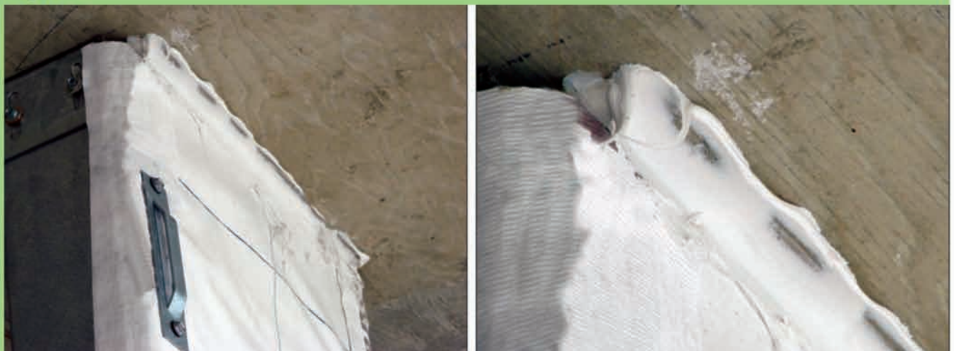
Close-up of the joint at a deflection track. Each façade layer must be built to accommodate the designed movement.
