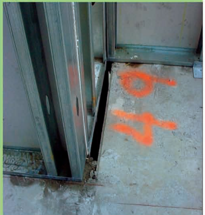
The dimensional inaccuracy of a cast-in-field concrete slab leaves an unexpected gap that may transmit fire and smoke.
