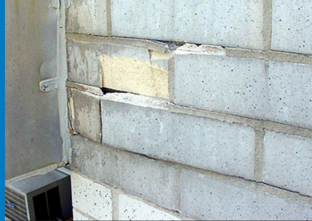
This photo depicts the disintegration of a sealed exterior wall surface in a heating climate (New York).
