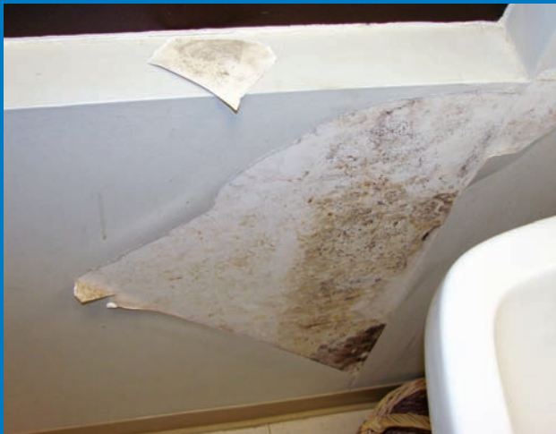
The disintegration of a sealed interior wall surface in a cooling climate (Alabama).
